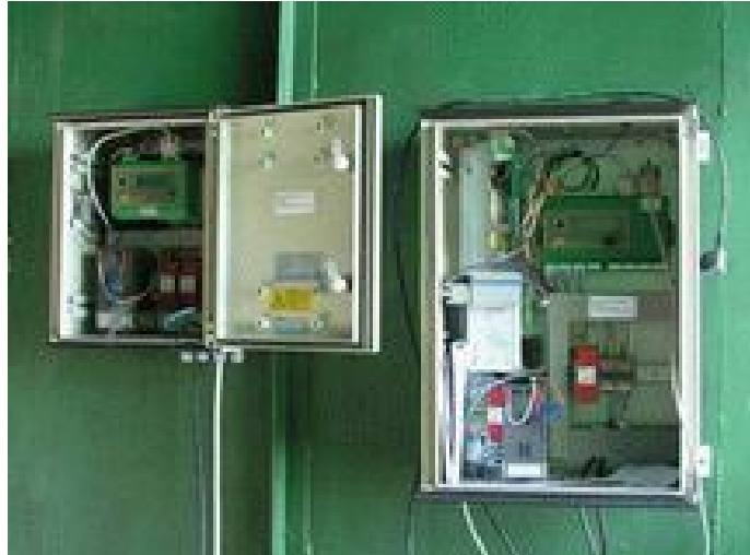
Figure 3: Arrangement of an automated gauge
