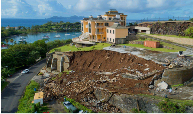
Figure 5: Landslide At Jax wall in Ratho Mill
