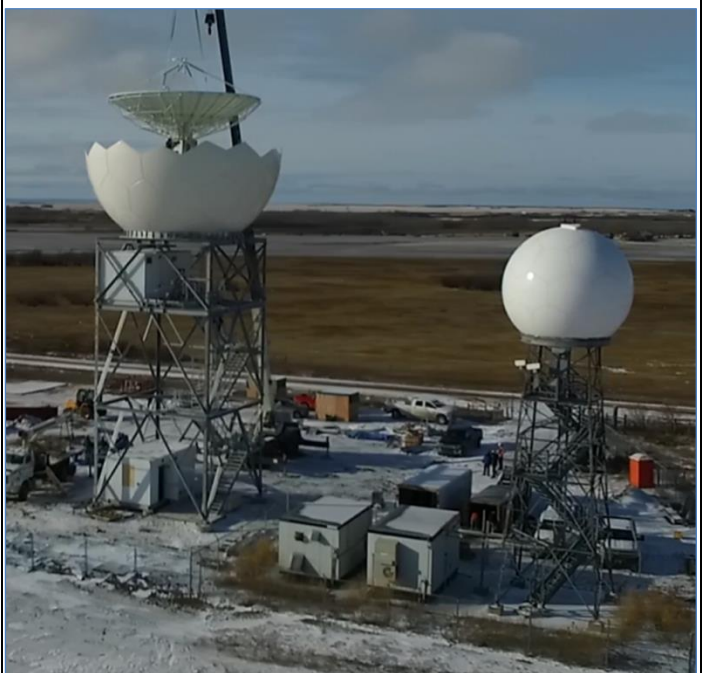
New S-band weather radar being installed at Radisson, Saskatchewan, Canada, alongside the C-band radar that the new radar replaces (Picture courtesy of Environment and Climate Change Canada)
