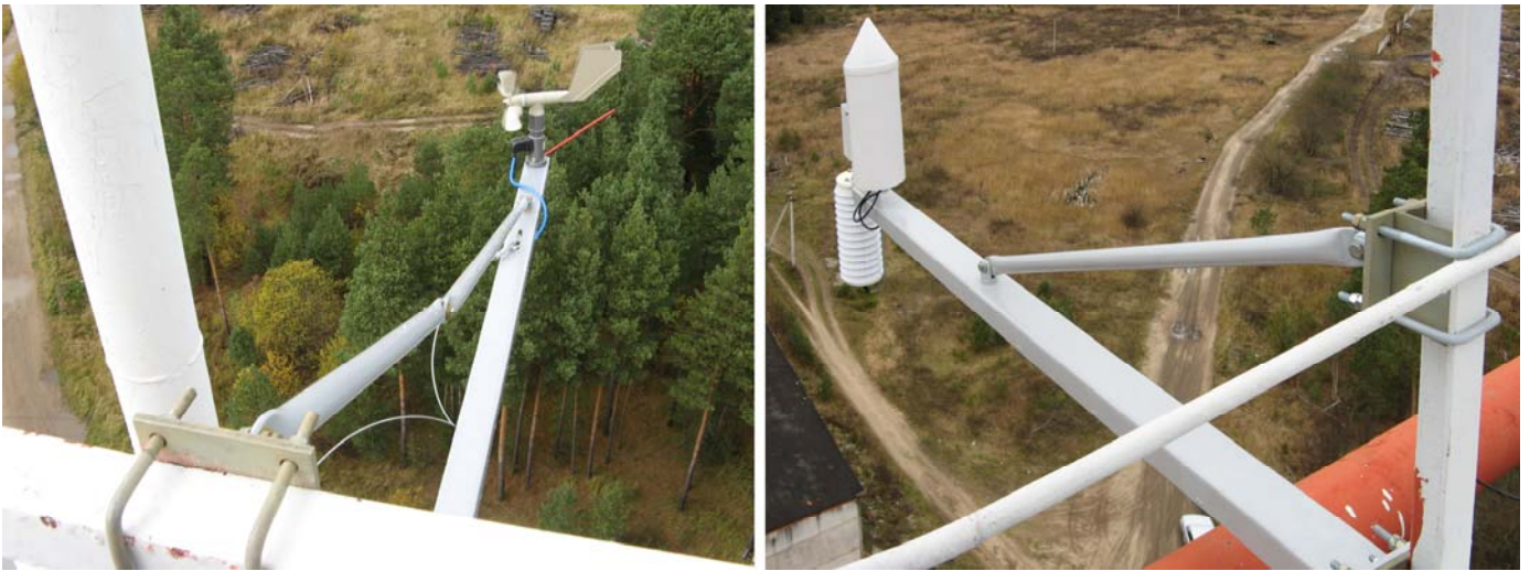
Figure 1 Wind speed and direction sensor, temperature and humidity sensor and precipitation sensor are placed on cellular communication tower
